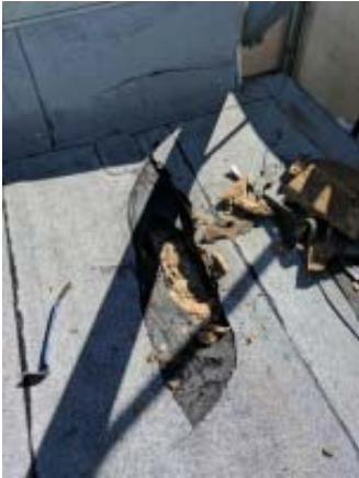
Roof damage on ARA building from ice, found by RENCO Roofing crew.
